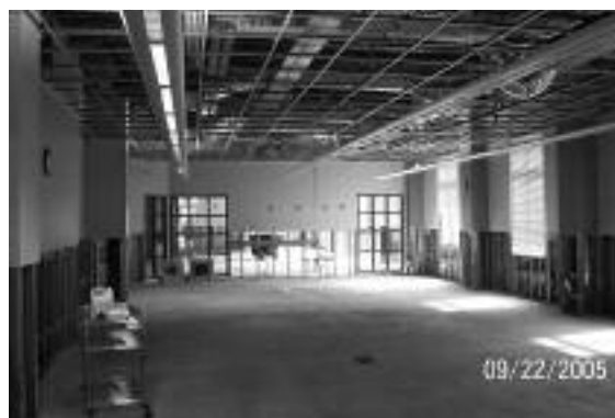
[Figure 5] Gutted first floor of the Gulf Coast Library at USM Gulf Park Campus.
